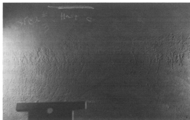
Fig. 11 Localized corrosive attack found in areas of certain liquid sulfur rail cars.
